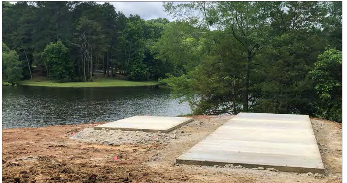
New 10' x 45' camper parking pads, plus new picnic pads and tables for 25 sites in Tishomingo State Park are nearing completion.
