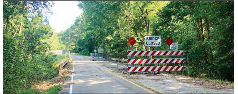
This bridge was reduced to one lane, allowing local access to a single homeowner.
