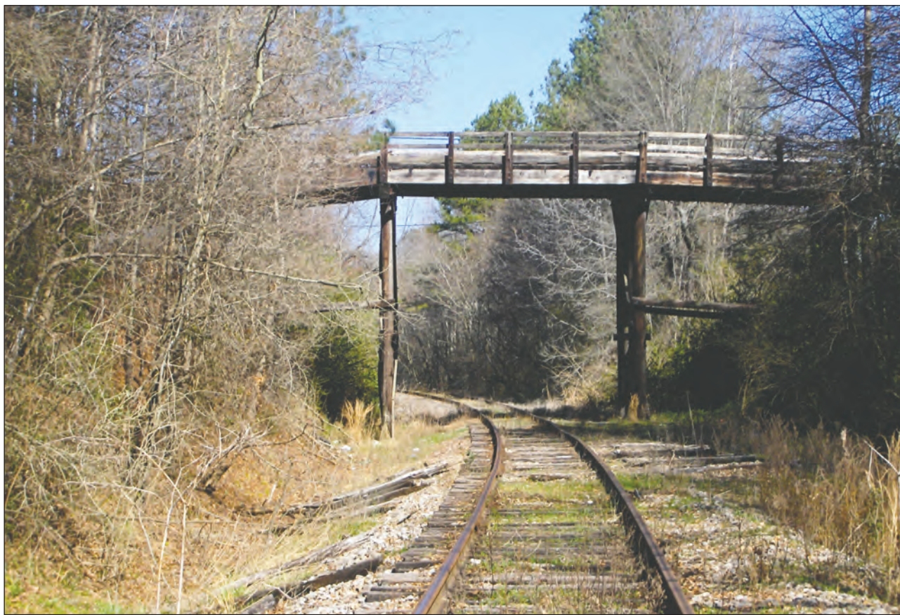
Railroad trestle bridge at Tishomingo. This one and another in Dennis were replaced with grade crossings in the last decade.
